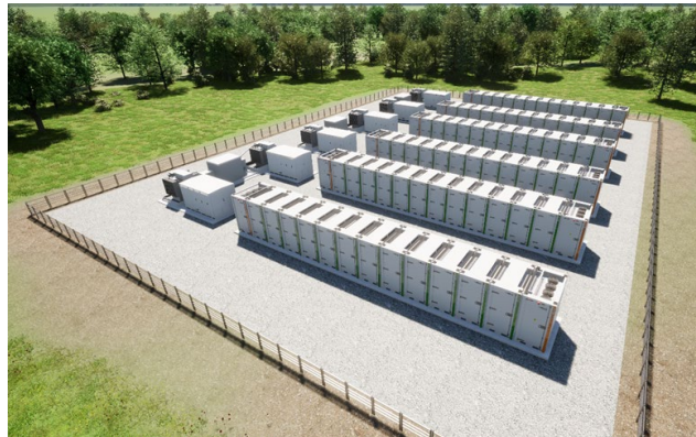
Battery Storage Compound
