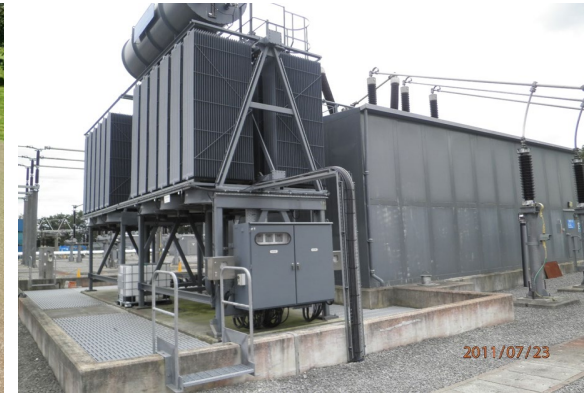
400 kV Power Transformer
